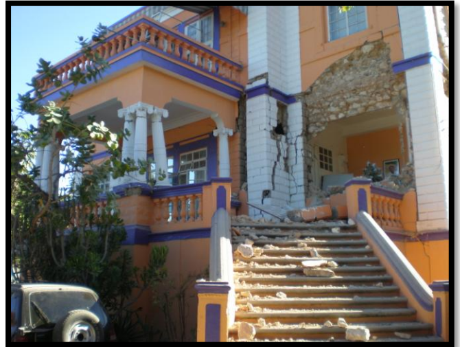
Fonkoze's severely damaged headquarters in downtown Port-au-Prince. Photo Credit: Leigh Carter
